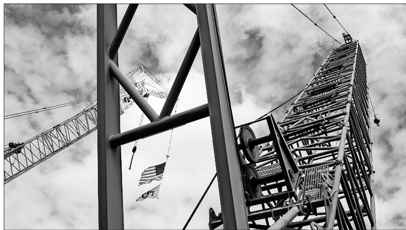
A crane used at the failed V.C. Summer Nuclear Station project was sold at auction for a fraction of its cost.
